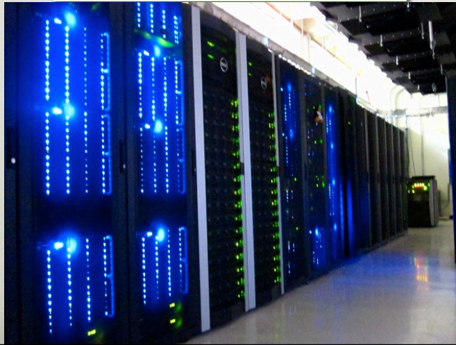
Machine room at Larson Hall
